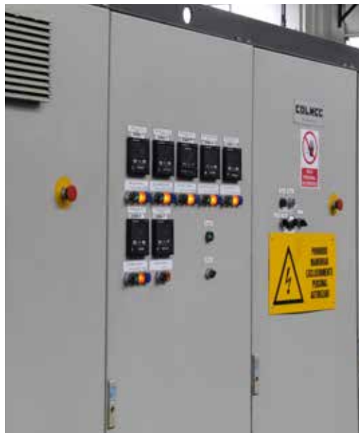
Switch cabinets for line control
